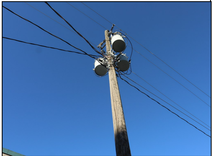
Photograph 8: View of a transformer located west adjacent to the site within the alleyway.
