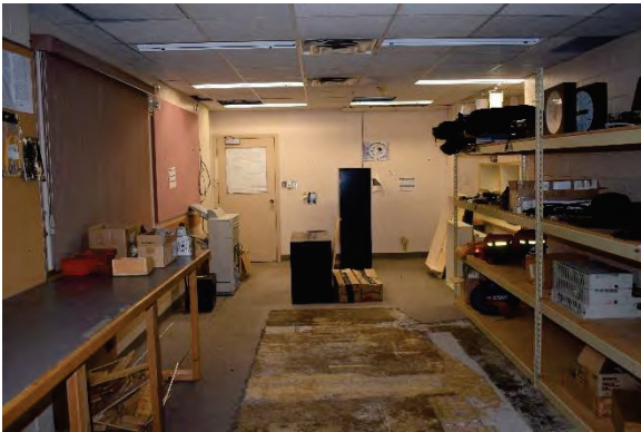
Photo 65: Storage room, representative photo
