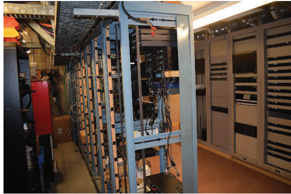
Photo 62: Server room, looking east
