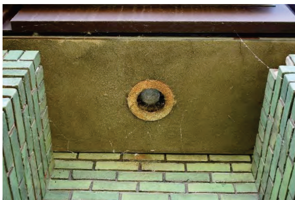
Photo 37: Recessed lighting fixture, looking south
