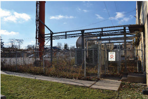
Photo 17: Tower base and equipment, looking west
