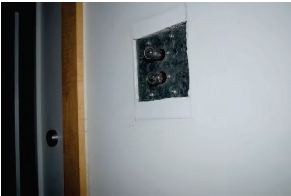
Photo 73: On Air/Off Air light, looking west
