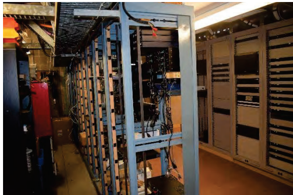
Photo 62: Server room, looking east
