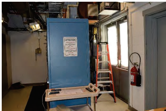
Photo 64: Transmission room, looking east
