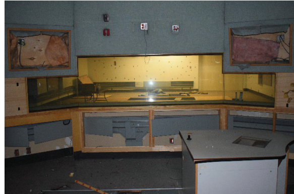
Photo 72: Control room, looking east
