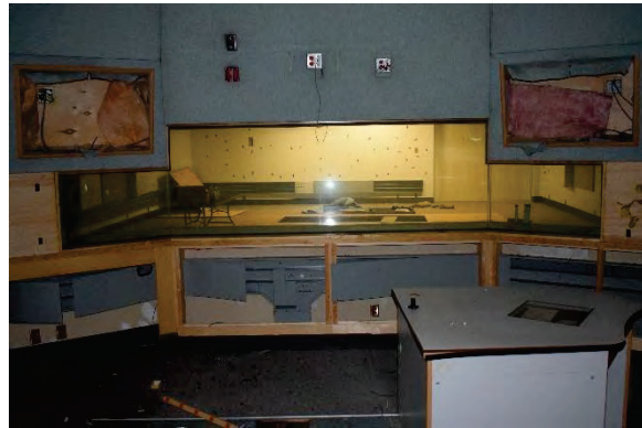
Photo 72: Control room, looking east
