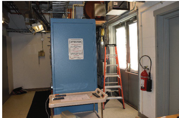
Photo 64: Transmission room, looking east
