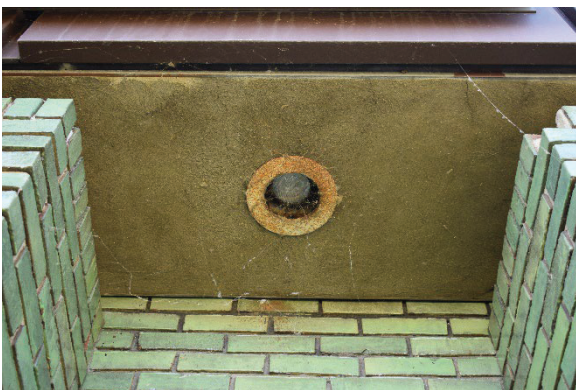
Photo 37: Recessed lighting fixture, looking south
