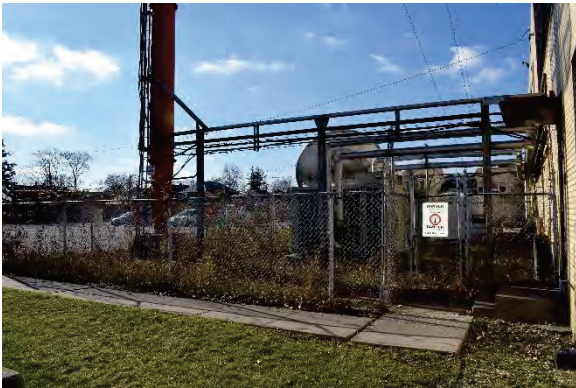
Photo 17: Tower base and equipment, looking west
