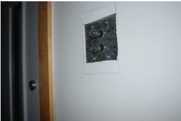
Photo 73: On Air/Off Air light, looking west
