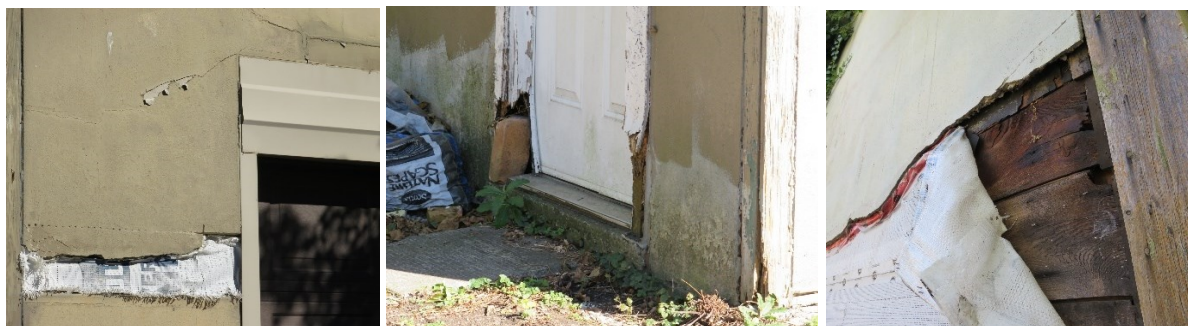
Damaged cladding, rotting wood, and cracks on the rear detached garage structure (photos taken by City Staff on October 8, 2025).
