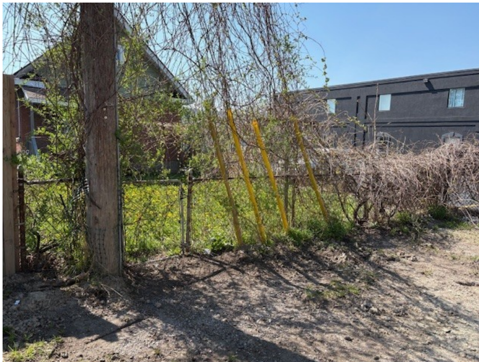
Figure 4 – Rear fence at 1526 Highland
