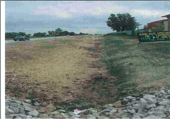
Photograph 1 ↑ No Name Drain/Parent Outlet Drain – West side of Banwell Road at Wildwood Drive, looking south
