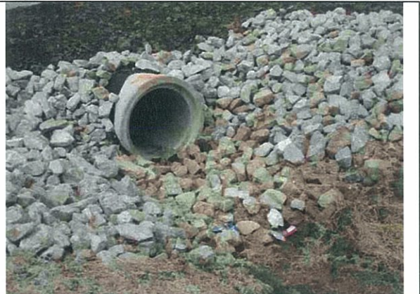
Photograph 2 ↑ No Name Drain/Parent Outlet Drain – West side of Banwell Road at Wildwood Drive, culvert dry
