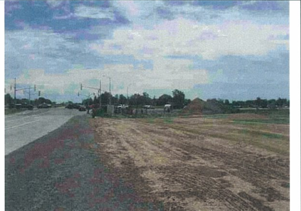
Photograph 4 ↑ Banwell Road – Looking south at EC Row Expressway, pit for tunnelling machine on northwest corner
