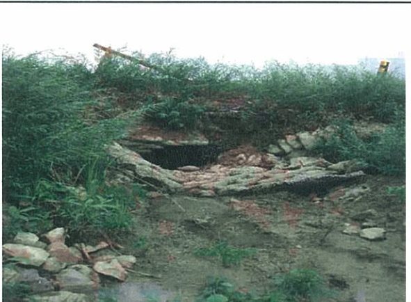
Photograph 16 ↑ Lachance Drain – West side of Banwell Road, collapsed road/culvert reinforcement
