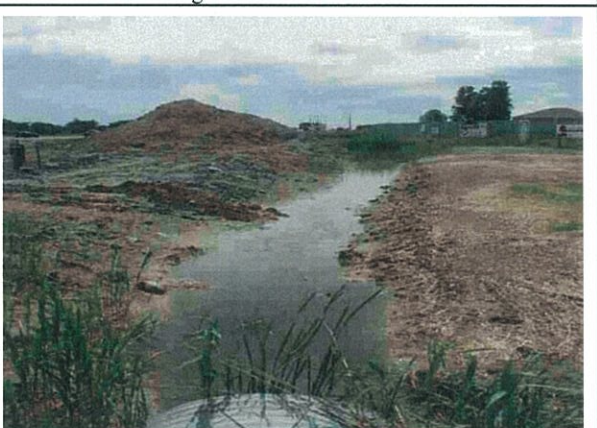
Photograph 6 ↑ No Name Drain – West side of Banwell Road, north of EC Row Expressway, standing water due to culvert blockage (see photo 8), culvert dry upstream in cattails
