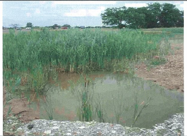
Photograph 8 ↑ Robinet Drain – East side of Banwell Road, shallow standing water, culvert under road partially blocked
