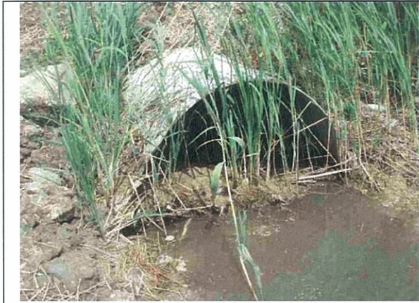
Photograph 7 ↑ No Name Drain – West side of Banwell Road, north of EC Row Expressway, culvert under Banwell Road blocked
