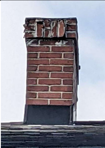
South chimney from east viewpoint. Widespread DIY mortar repair; visibly cracked bricks; missing ricks from soldier course; warped chimney crown.
