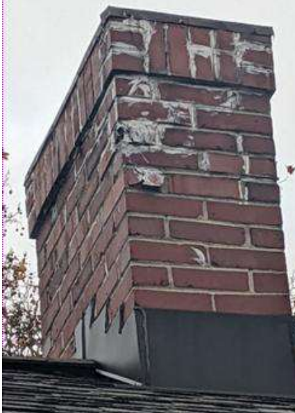
South chimney from NW viewpoint. Widespread DIY mortar repair; visibly cracked bricks.
