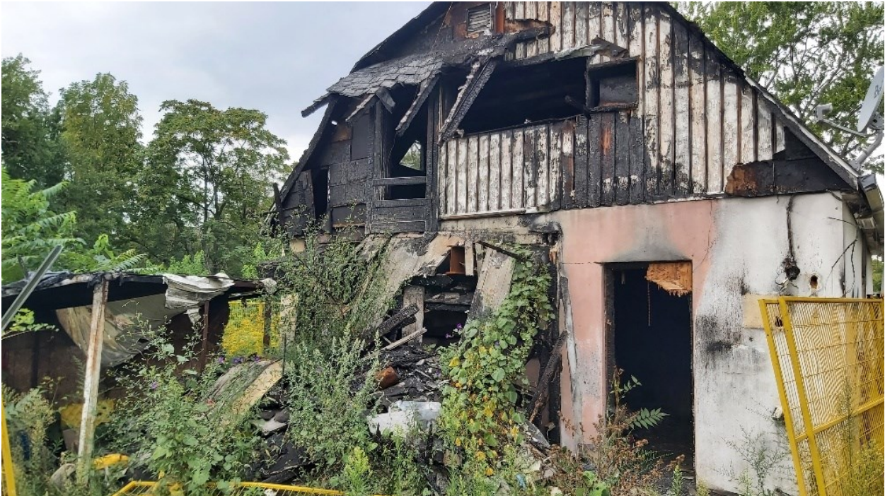
Subject Site, Fire Damaged garage
