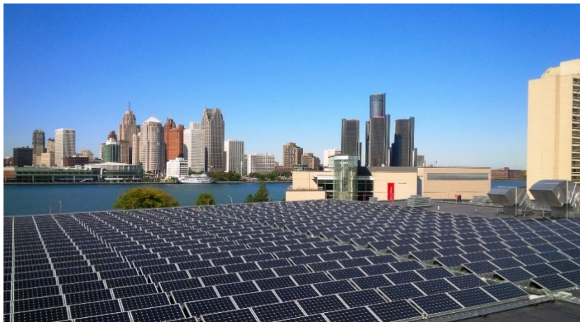
Figure 24: Solar PV Installation – Windsor International Aquatic Centre
