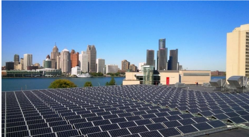
Figure 24: Solar PV Installation – Windsor International Aquatic Centre
