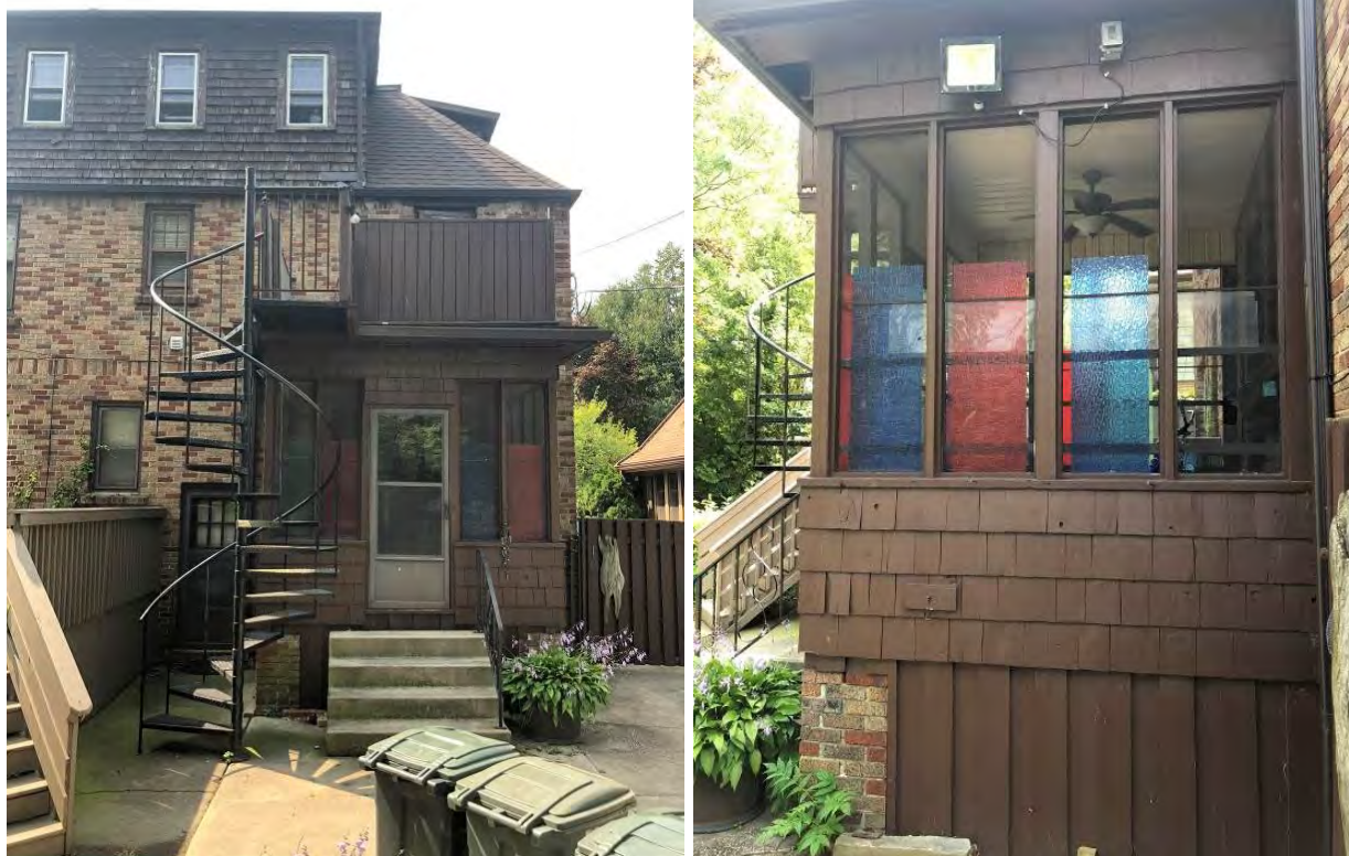
View of rear attached enclosed porch and fire escape staircase which is to be removed.
