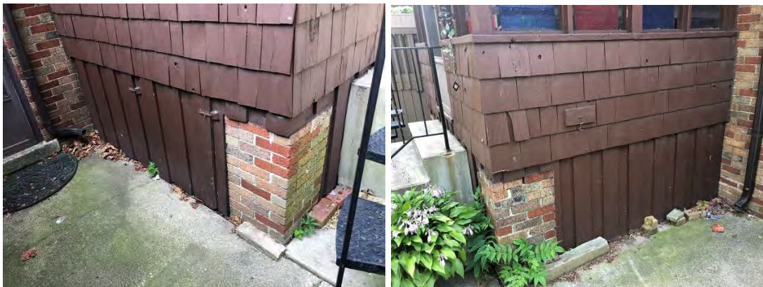
Similar brick used on both exterior facade of main building and pilings for the rear enclosed porch.
