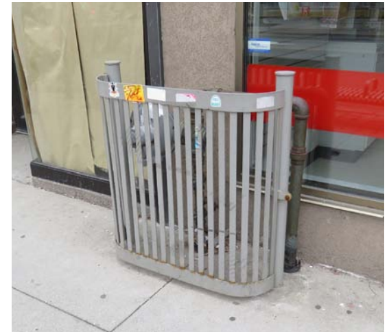
Figure 39. Site mechanical equipment at rear if possible instead of along the front facade
