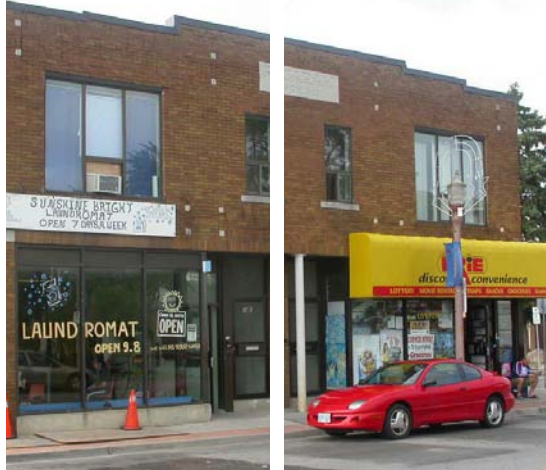
Figure 37. Window on the left is open whereas on the right it is blocked with signs
