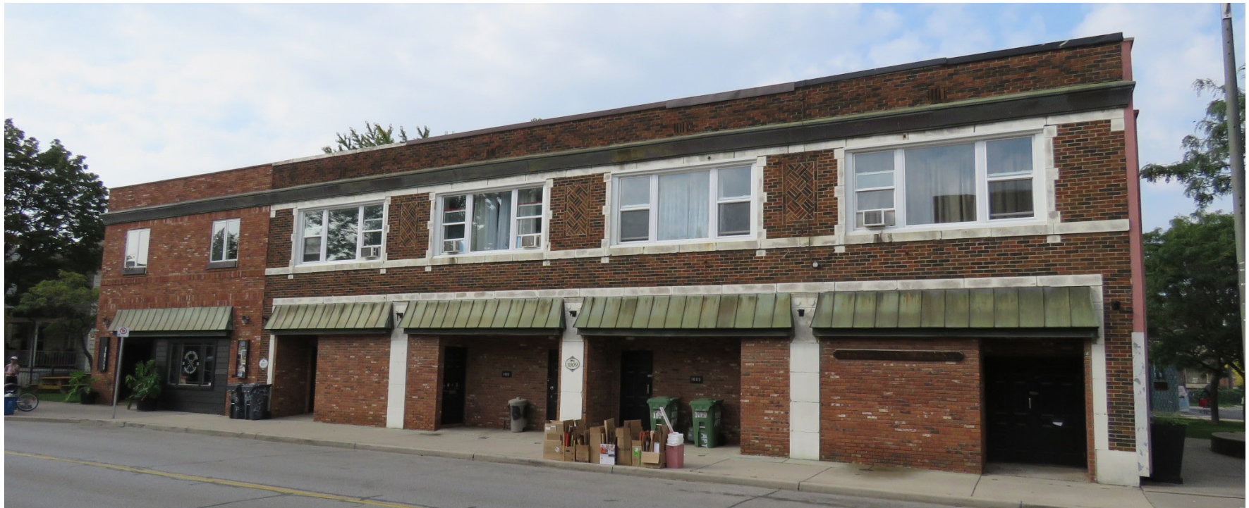
Figure 106. A building facade on the west side of Drouillard Road with original storefront windows and doors bricked in, eliminating the connection with the street
