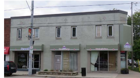
Figure 135. Original brick material has been painted over
