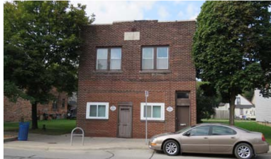
Figure 111. Example of a traditional commercial building that has doors and windows bricked in and replaced
