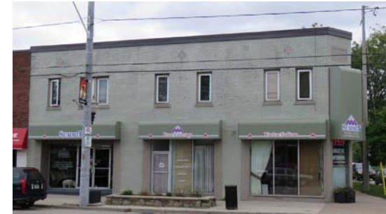
Figure 135. Original brick material has been painted over
