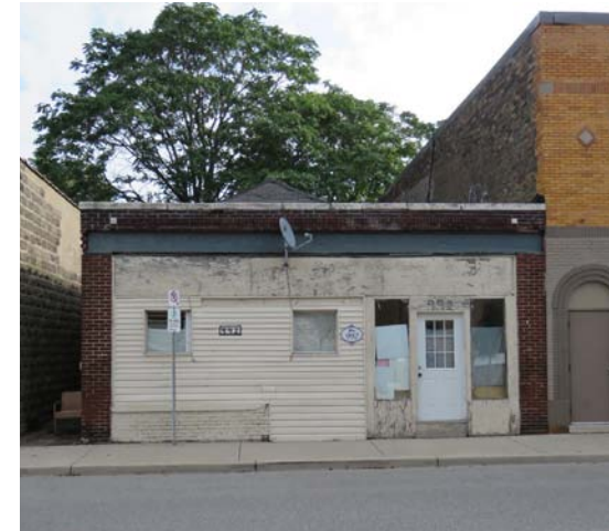
Figure 108. Example of a building in Ford City where storefront doors and windows have been boarded up
