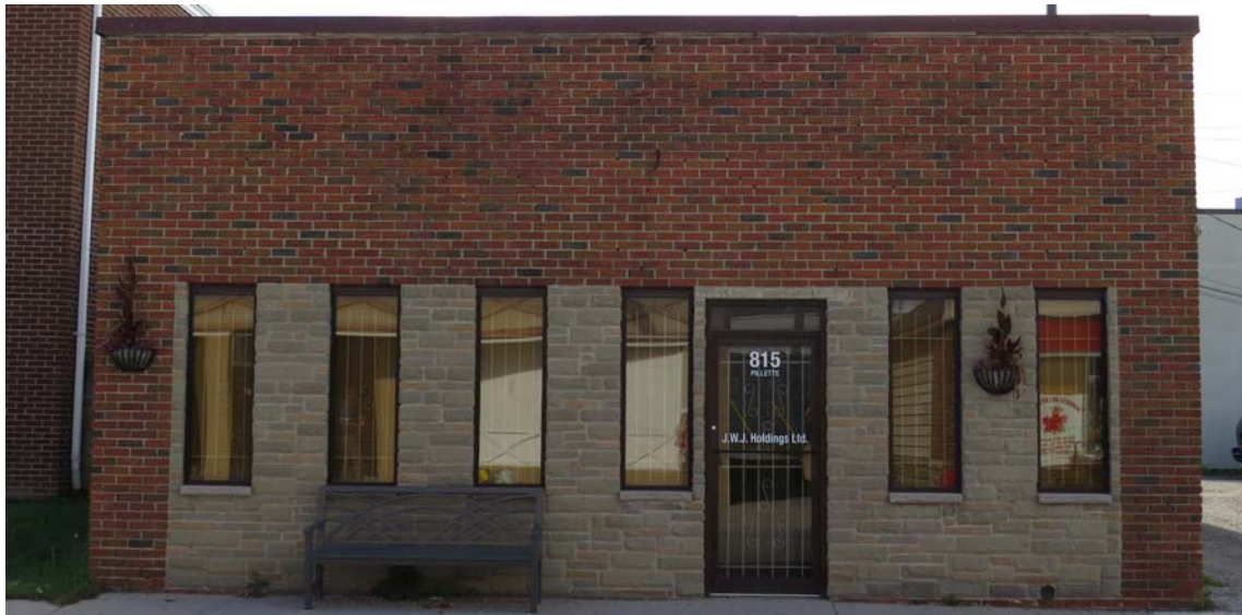
Figure 127. Windows have been removed and non-traditional materials fill in the original traditional Main Street storefront at 815 Pillette Road
