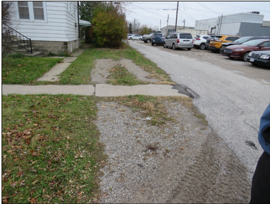
Figure 8 - Looking west towards 2321 George Ave driveway and driveway approach partially in Alley
