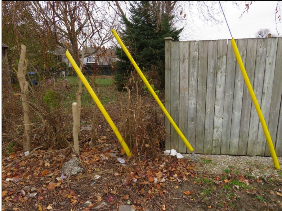
Figure 5 - Looking south at guy wires and anchors in Alley (2321 George Ave on left)
