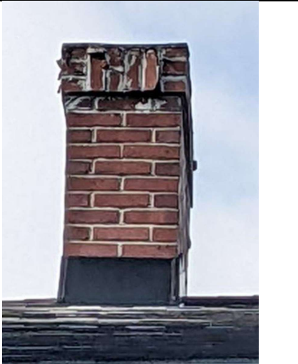
South chimney from east viewpoint. Widespread DIY mortar repair; visibly cracked bricks; missing ricks from soldier course; warped chimney crown.
