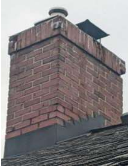
North chimney from SW viewpoint. More missing soldier-course bricks and cracked bricks; mortar erosion just above flashing. No visible cement or metal chimney crown, not offering any water protection.
