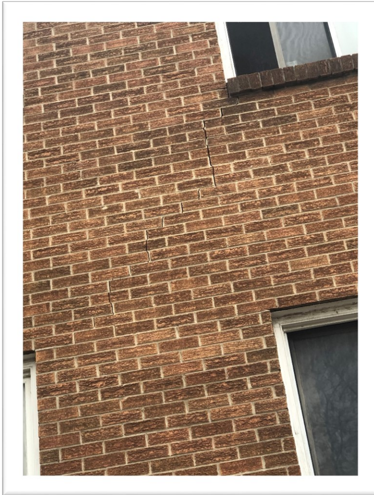
Repair cracks in exterior walls and foundation
