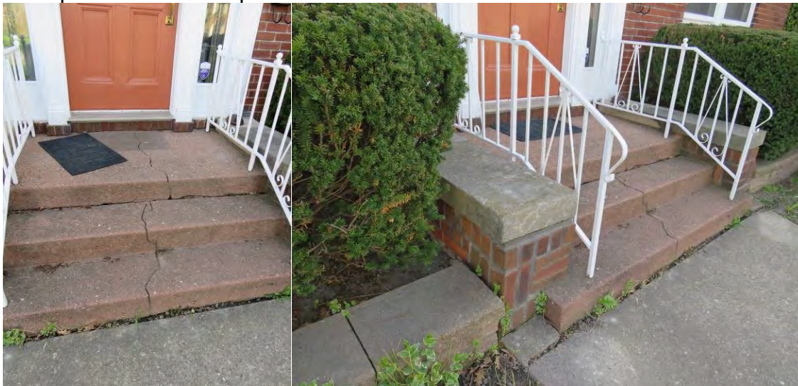
2022 photo of the front porch and visible center crack
