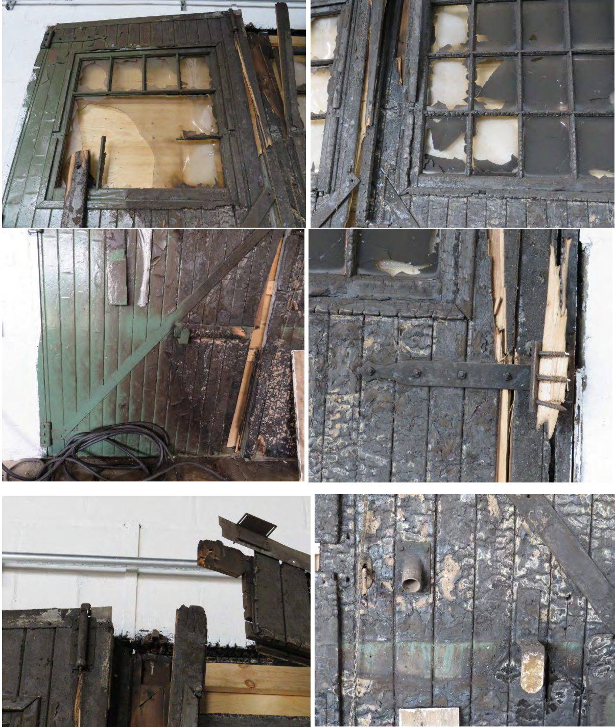
Close-up details of the fire damage to the interior of the wood doors, photographed by Administration in February 2022
