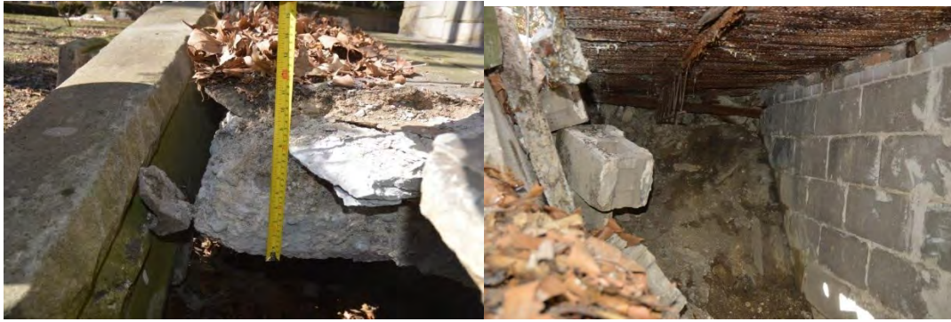
View of hole at slab and view underneath porch with no backfill (Source: Jesse Garant)
