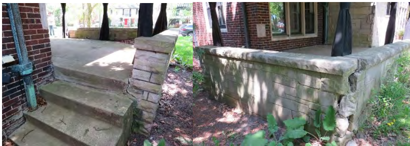
On left, back steps leading to front porch. On right, the exterior southwest corner of the porch wall.
