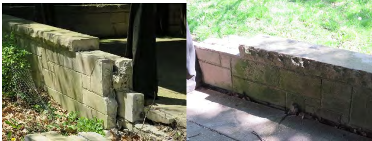
View of porch wall still standing with stone coping and veneer stone pieces on the interior and exterior sides.
