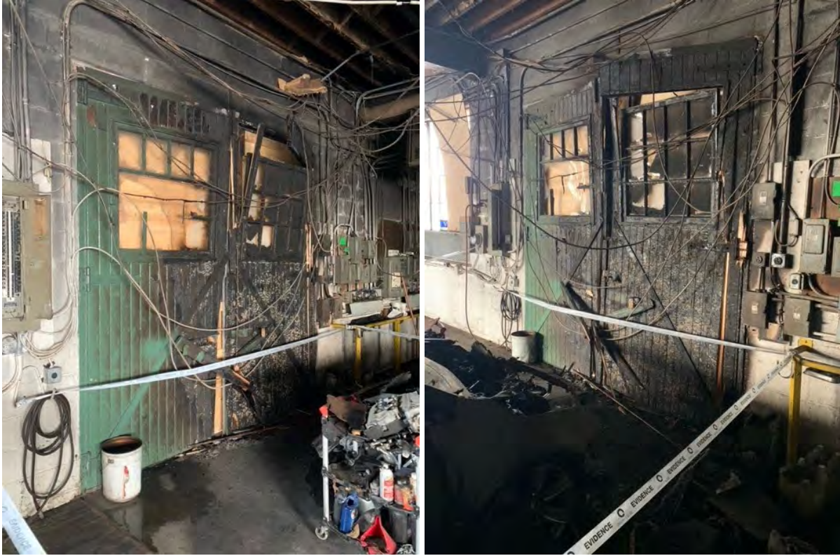
Interior of the wood doors immediately following the work shop fire, photographed by owner in January 2022
