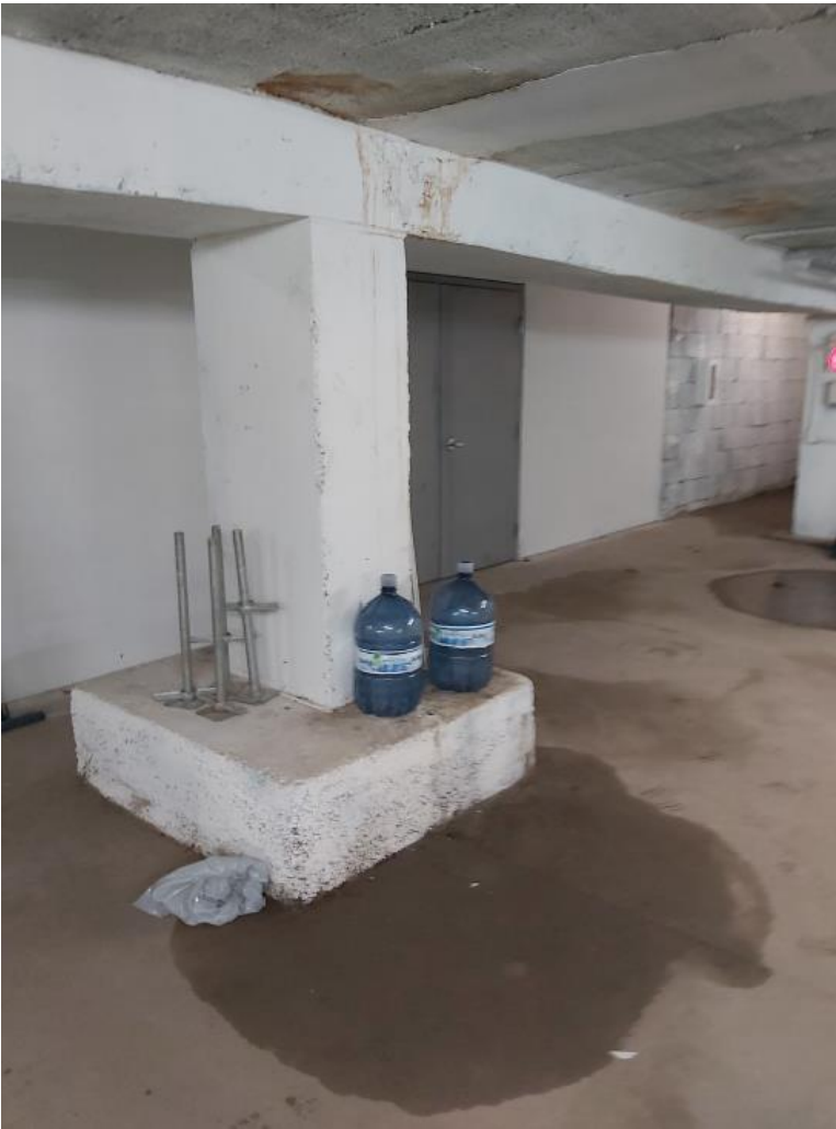
5. Water infiltration in underground parking garage.
