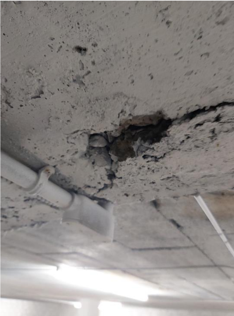
7. Close up of affected concrete structure.
