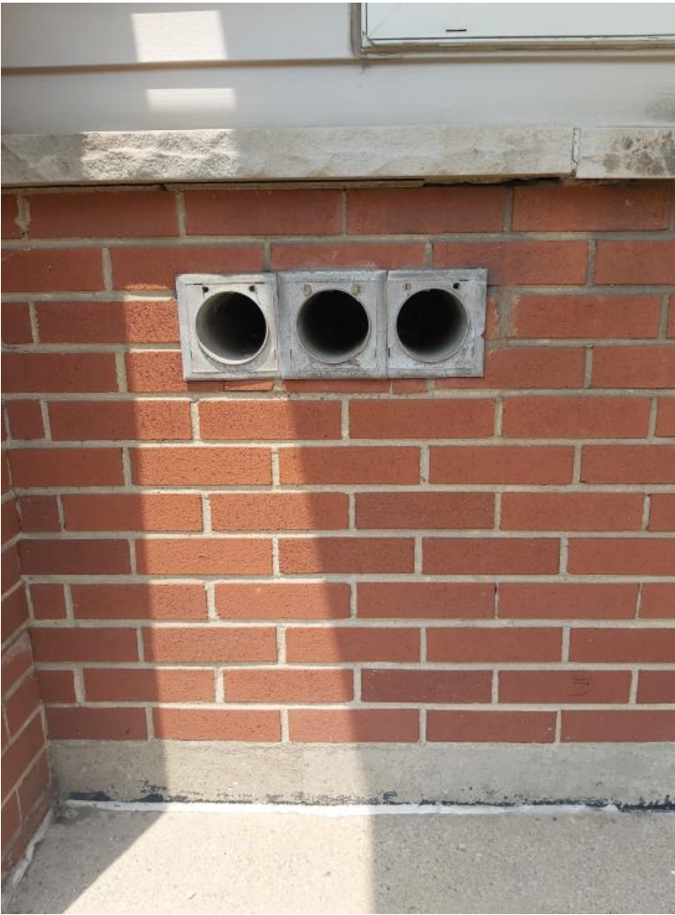
13. Missing / defective grilles.
