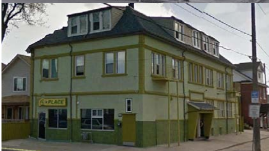
Figure 66. EIFS is an undesirable building material that is often used to cover brick
