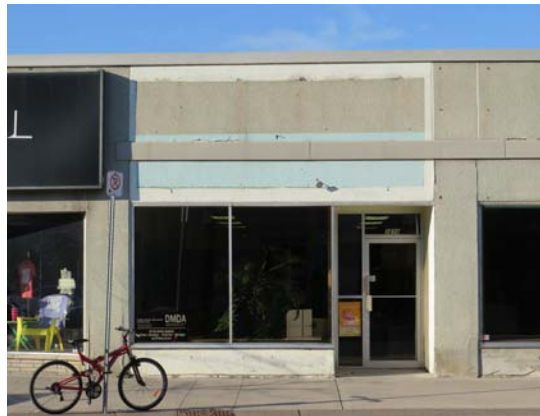
Figure 149. A traditional Main Street building facade that is covered with non-traditional materials and is missing signage
