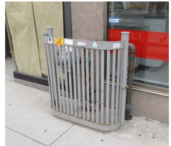
Figure 38. Site mechanical equipment at rear if possible instead of along the front facade
