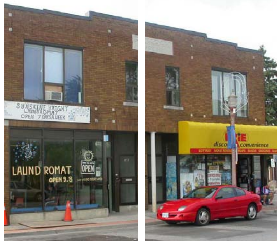
Figure 36. Window on the left is open whereas on the right it is blocked with signs
