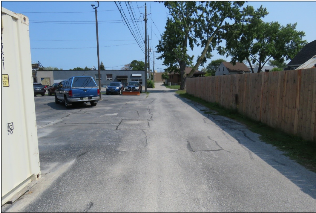
Figure 3 - Looking east from west end of portion of alley requested for closure
