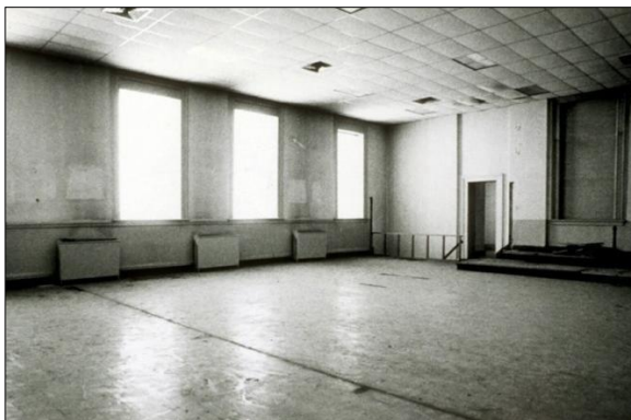
Interior Court Auditorium – blocked in windows and lowered ceiling to accommodate air conditioning ducts c1981 (E. McLean)
