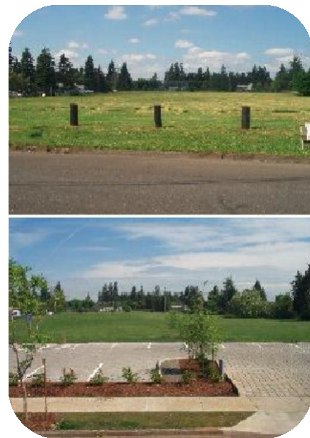
Figure 2: Before (above) and after (below) East Holladay Park porous parking lot construction (City of Portland, 2007)
